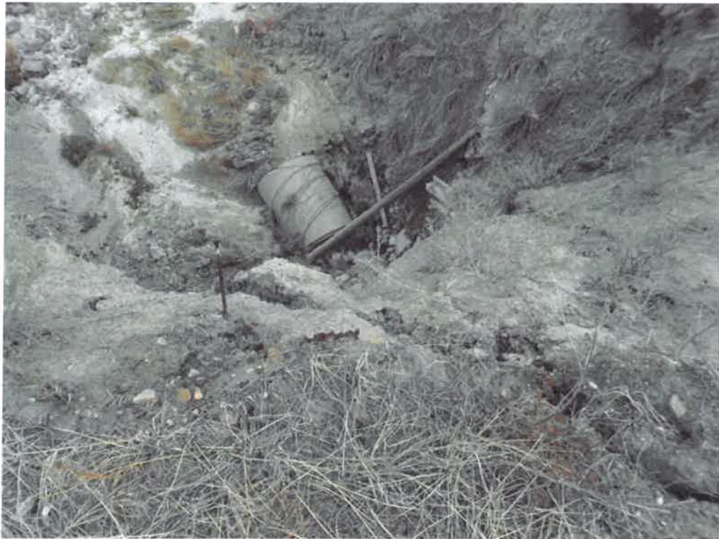
Looking down washout #3
