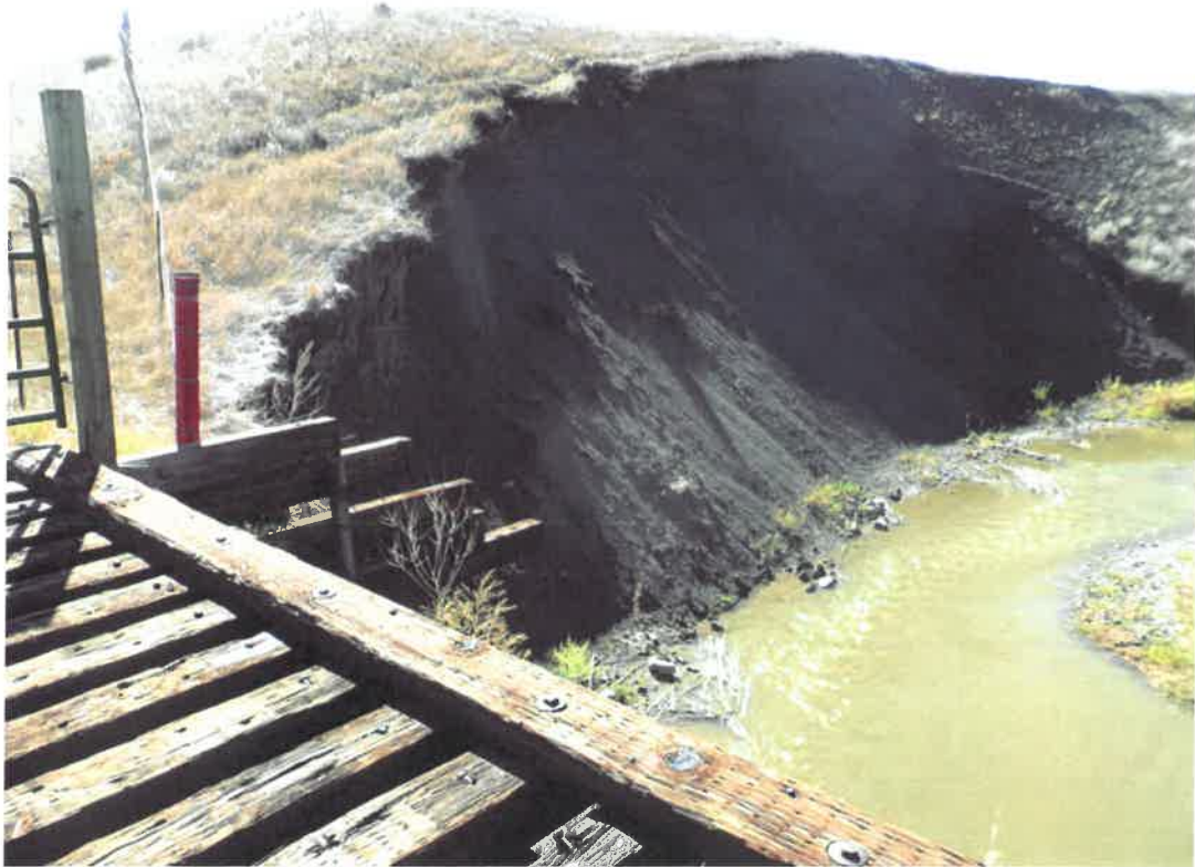
Bridge #23 being undercut by Rapid Creek.
