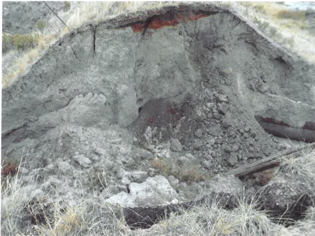
Inside Badlands National Park Washout #2
