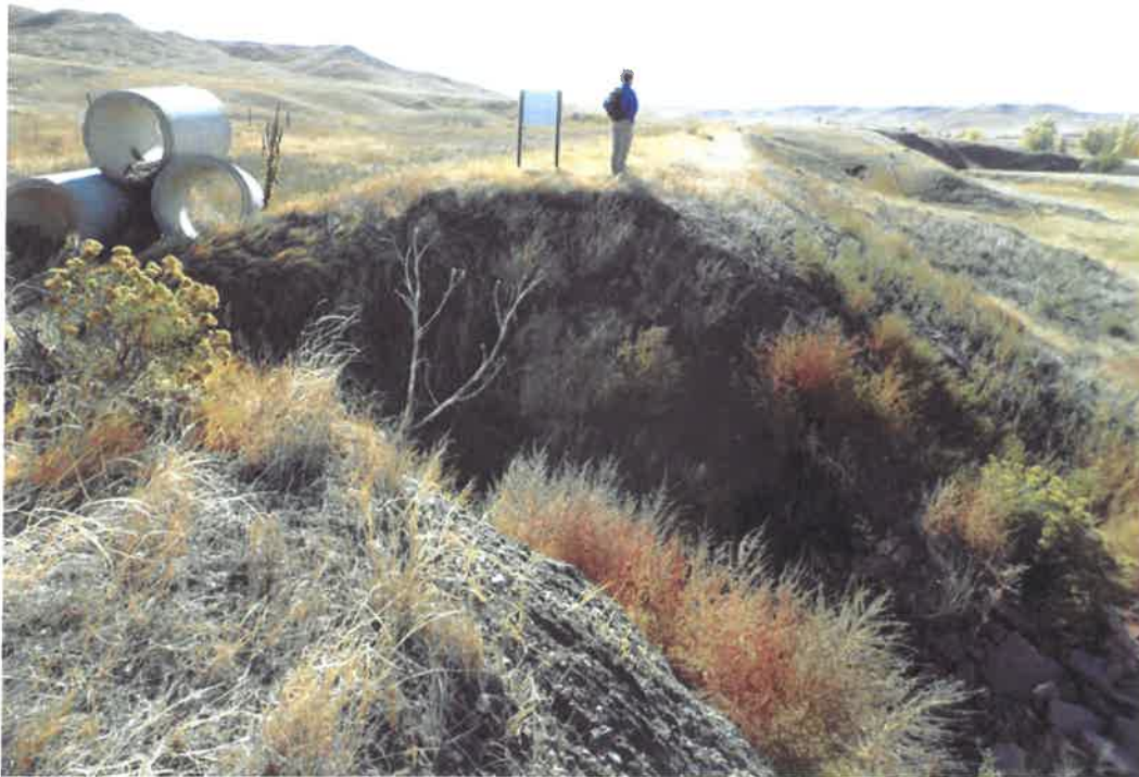
Washout just east of the Cheyenne River Bridge
