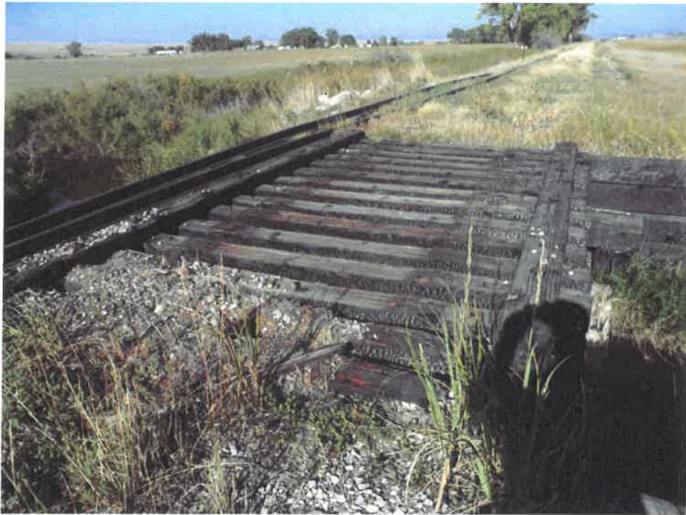
This bridge has been scorched by fire
