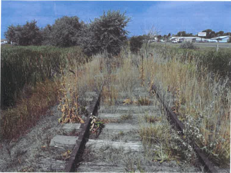
Railroad corridor just west of St. Patrick's Street. Notice rails and ties still in place.
