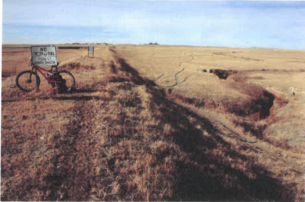
A route around the washout to the right in this picture (north side) can be maintained on railroad property if money cannot be found to fix the breach. The top of the washout is located behind the bicycle in this picture
