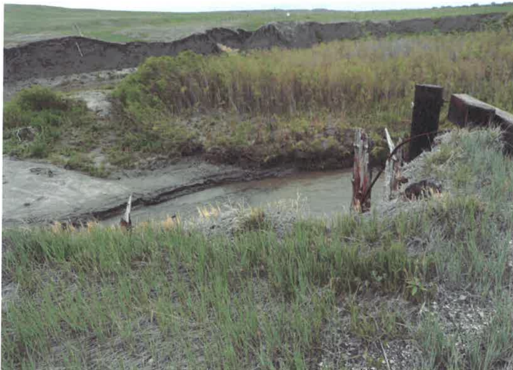
Bridge #24 washed out and completely gone.
